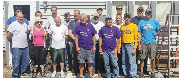
Members of the Love INC Home Repair Ministry and Kohler Co. Model Shop staff members recently pitched in to help upgrade Neighbor Mary's windows to meet city code.
